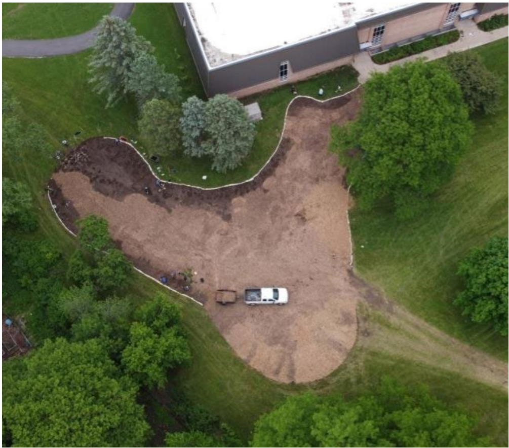
Aerial photo (right) of site for Glen Hill's new outdoor gathering and garden space.
