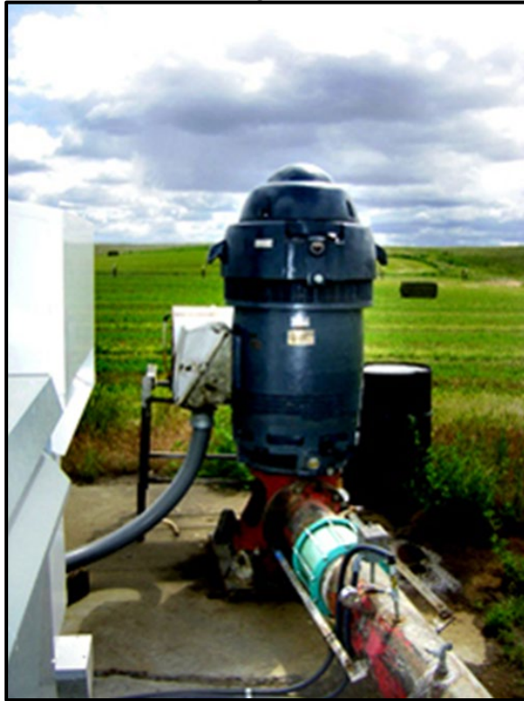
Figure 12-34: Water Well Pump Powered by Electric Motor, Washington
