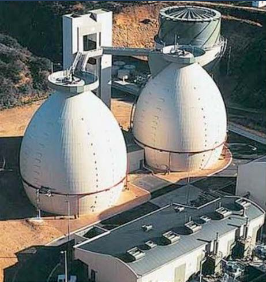
Wastewater Treatment Plant (WWTP) Digester in Boston MA
