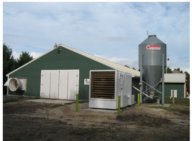
Scrubber is attached to the side wall fan of poultry house to remove pollutant emissions to improve air quality.
